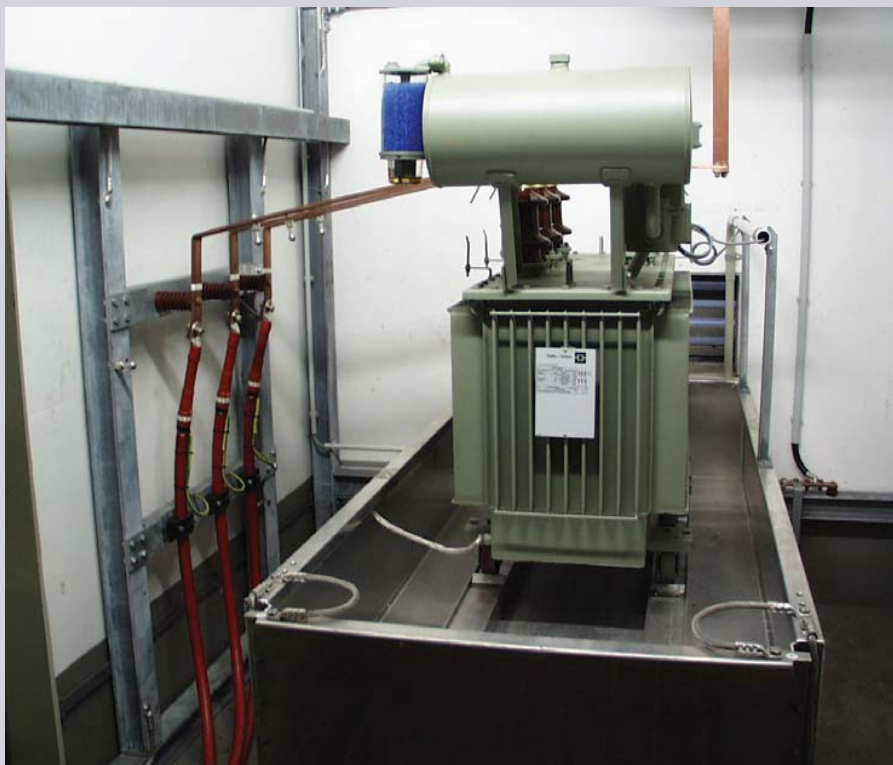
Neutral earthing transformer
